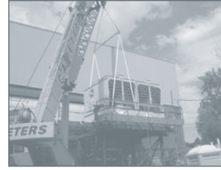
HVAC equipment being delivered in May, 2010
