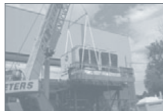
HVAC equipment being delivered in May, 2010
